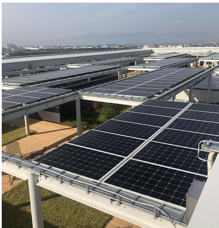
Solar Panels on the Rooftop. Lake Biwa Can Be Seen in the Distance.
